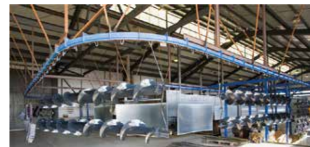
Powder paint installation
